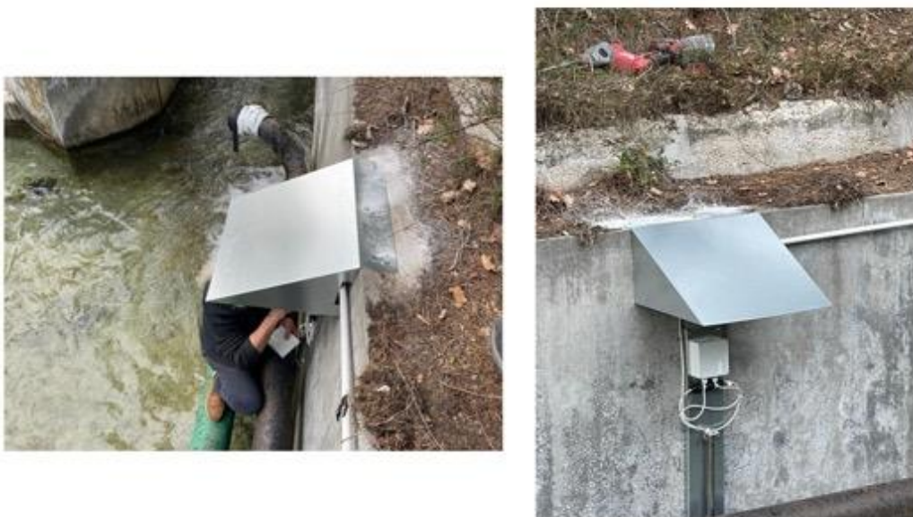
Roof installed on February 26 th at Giardino spring (site 8) to protect the transmitter unit
