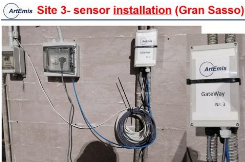
Figure 3.16: Installation logistics of the site 3 (SW Gran Sasso groundwater intake tunnels): gateway location.
