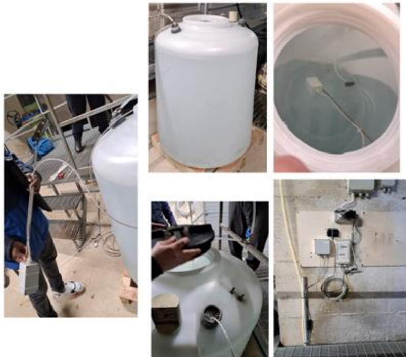
Figure 3.23: Sensor prototype installation characteristics of site 2 (NE Gran Sasso groundwater intake tunnels).
