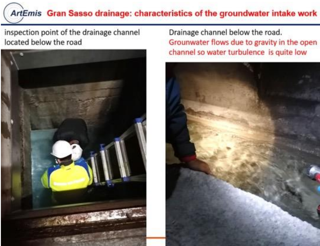
Figure 3.6: Gran Sasso drainage through channels located below the highway road tunnels.
