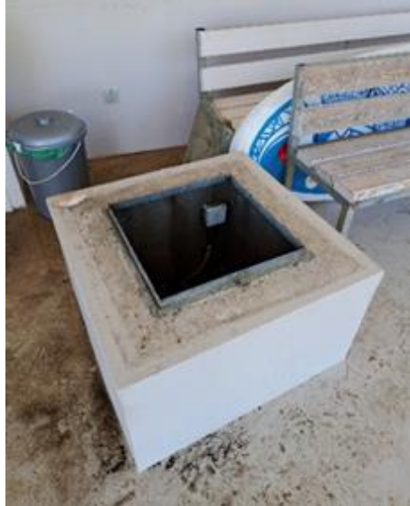
Figure 2.5: The installation well of the Brunello Station (System Number 4).
