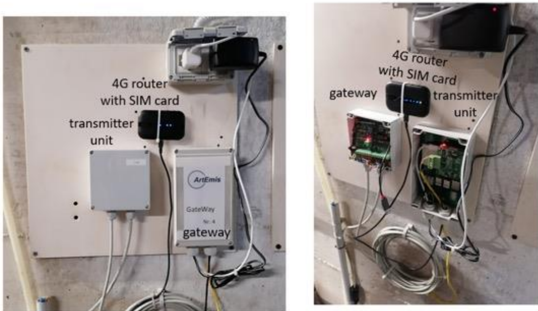
Figure 3.9: Installation logistics of the site 2 (NE Gran Sasso groundwater intake tunnels): transmitter unit and the gateway.
