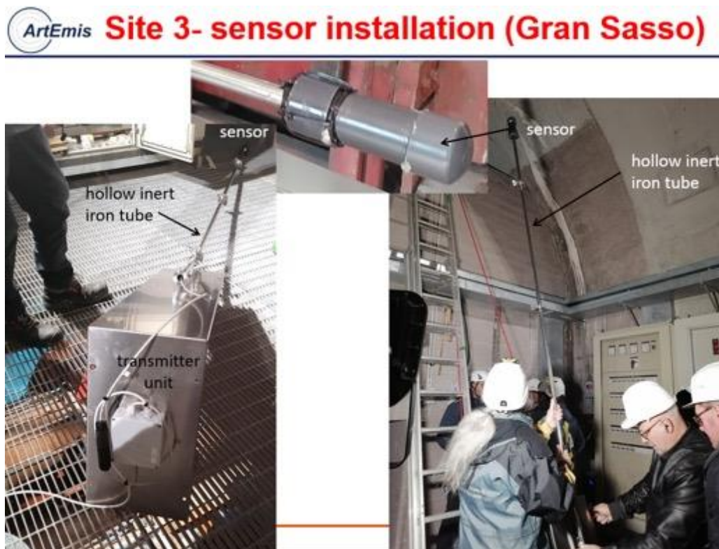
Figure 3.14: Installation logistics of the site 3 (SW Gran Sasso groundwater intake tunnels): installation activity.
