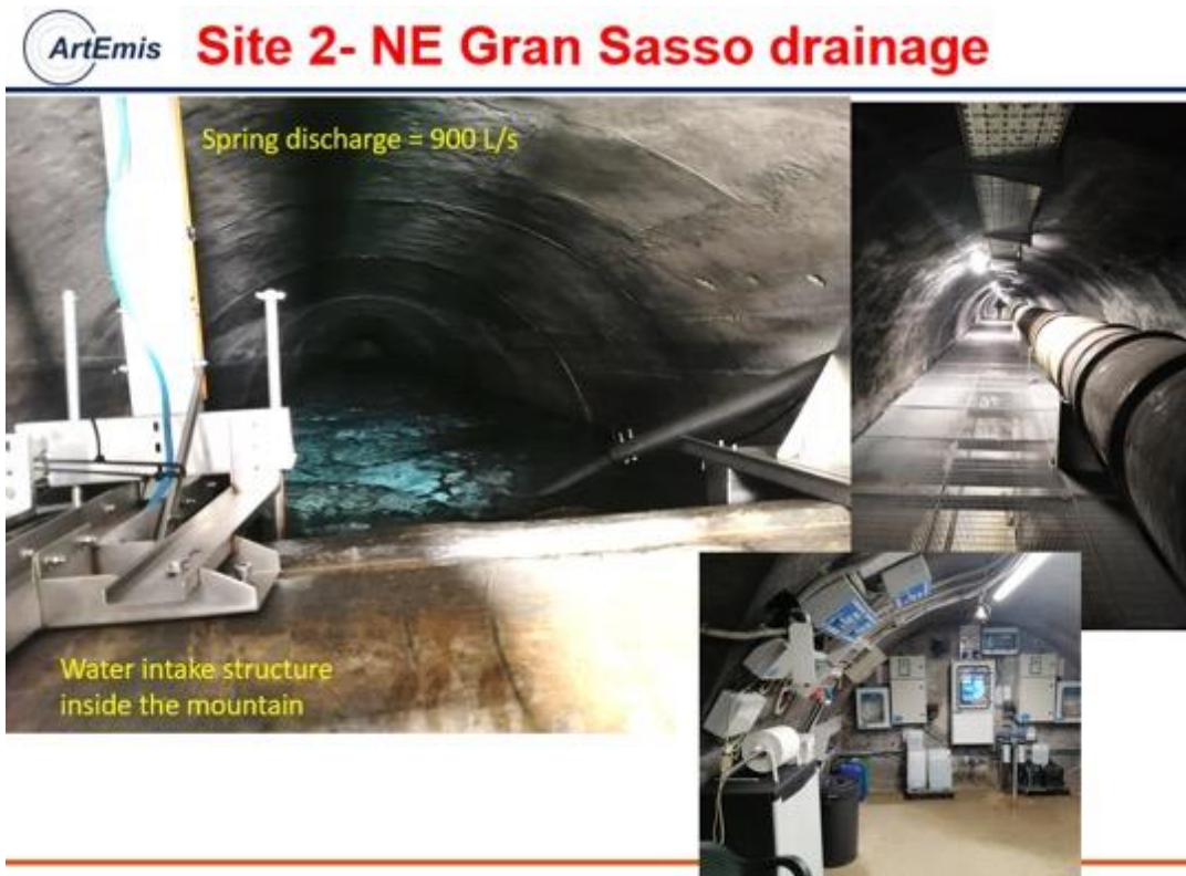
Figure 3.7: The ending part of the NE Gran Sasso groundwater intake tunnels (picture on the left) and the related hydraulic works (aqueduct – picture on the top right – and control room – picture on the bottom right).
