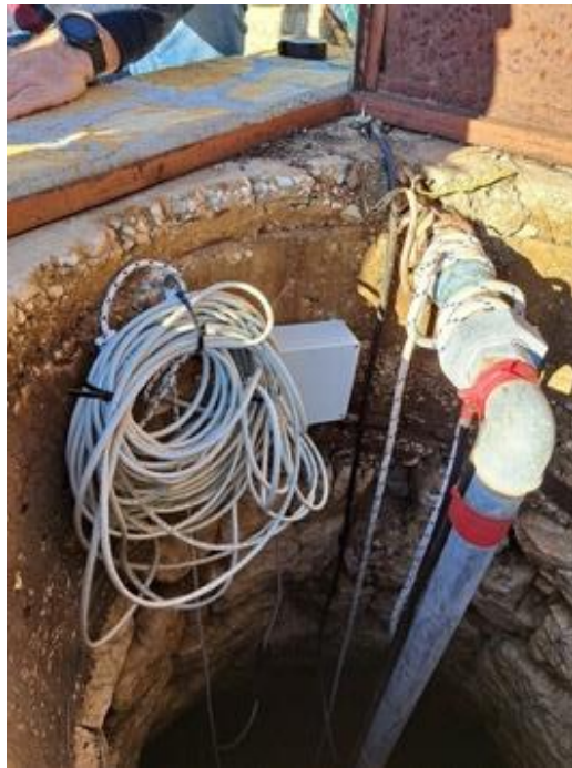
Figure 2.15: Transmitter unit of Komilio Station, as it was mounted onto the walls of the well.
