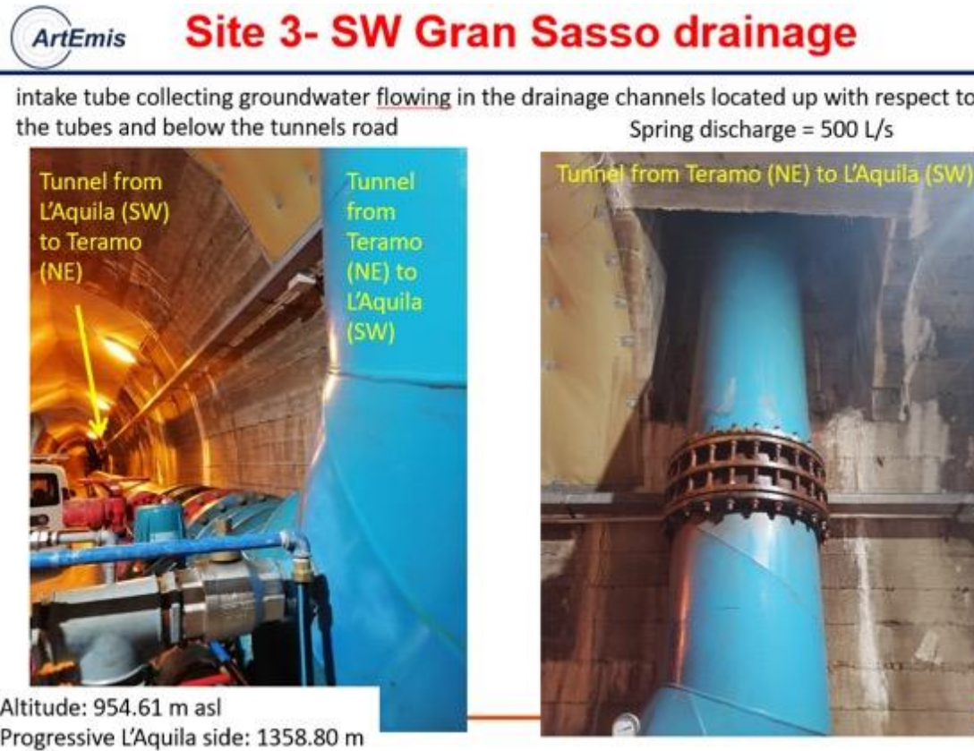
Figure 3.12: The site 3 (SW Gran Sasso groundwater intake tunnels): vertical tubes capturing groundwater from the above intake channels. The last are placed just below the highway road Gran Sasso tunnels.
