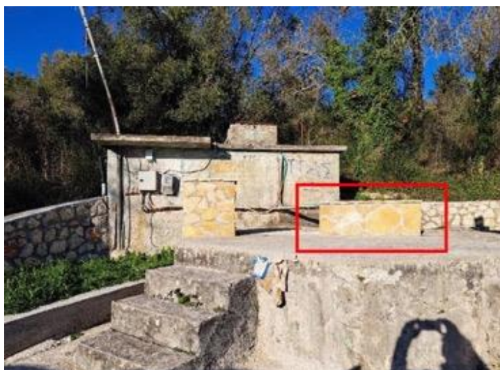
Figure 2.11: Installation site of the Komilio Station (System Number 5).
