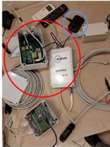
Figure 2.10: The gateway unit (denoted inside the red circle) and the D-link router (denoted by the light blue circle) used for the installation of Brunello Station.
