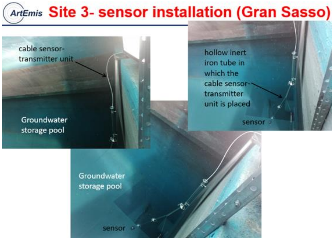
Figure 3.15: Installation logistics of the site 3 (SW Gran Sasso groundwater intake tunnels): the sensor prototype was placed in the accumulation piezometric tank of the water hydraulic work.
