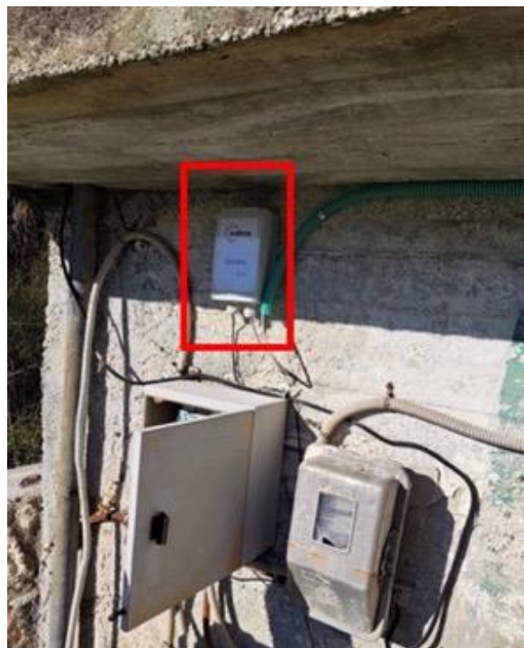
Figure 2.16: Gateway (base) unit of Komilio Station, as it was mounted onto the walls of the well (red rectangle), and the power supply system of installation site.
